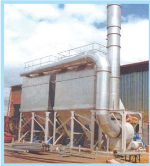
Fume extraction from hot-dip galvanizing process
