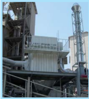
Cement Plant / Belt Conveyor Process, Cement / Lime industry
