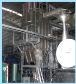
Waste gas cleaning for garbage disposal plant separating of dust and sulphur dioxide
